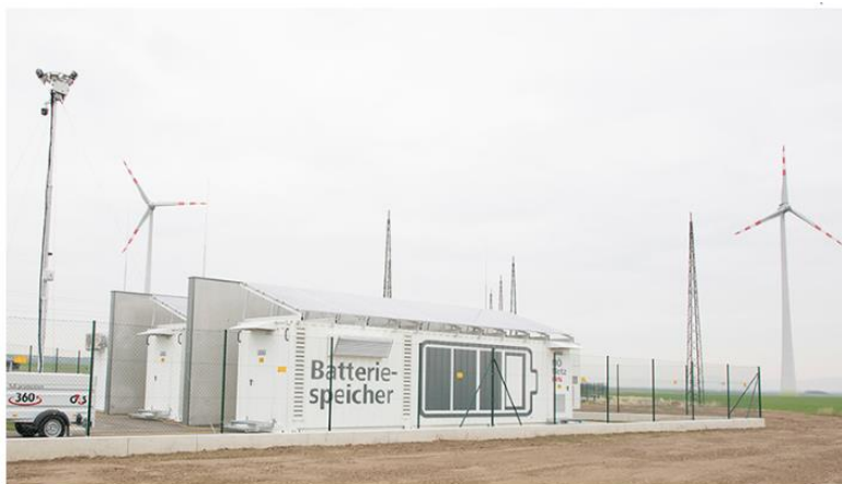
Figure 7 – Battery storage integrated to EVN wind farm in Prottes, Austria (noeORF.at, 2019)
