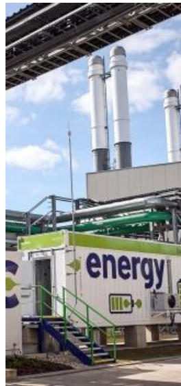
Figure 12 – C-Energy battery storage and the Plana power plant (C-Energy)
